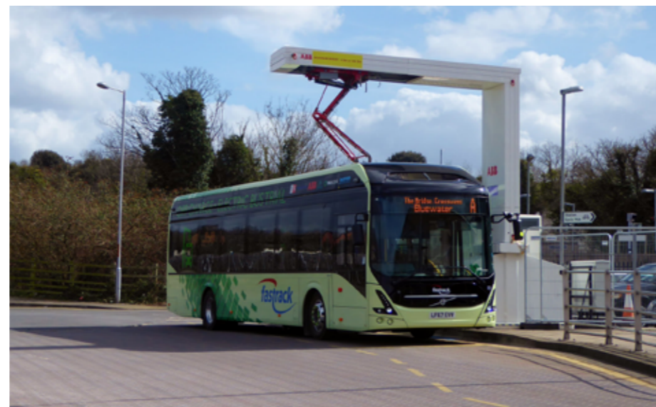
Fastrack Electrical Bus Charging Facility.
